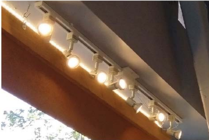
Lighting Fixture with new LED lamps.
