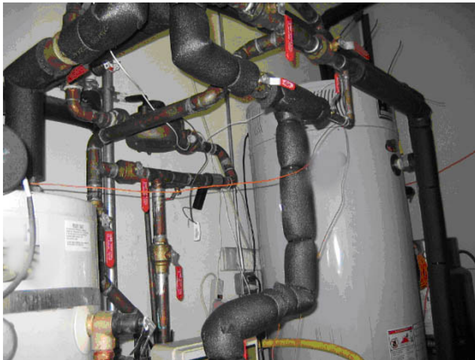
Figure 4. Water heaters installed for monitoring
