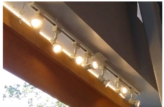
Lighting Fixture with new LED lamps.
